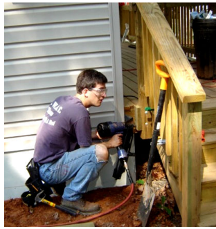
Nate got creative in filling in a "hole" in the railing.
