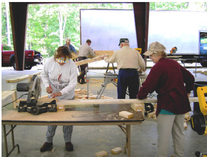
An "assembly line" was set up to cut and sort lumber and then assemble the bunks. Dawn and Esther were "cutters" for the day.
