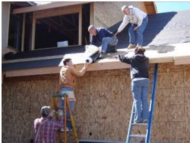
Jim, and the Blakeman's help Harley install the "ice shield" strips on the new addition to the Golden Bell Camp lodge
